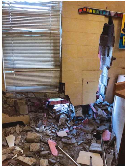
08/10/21- Interior classroom damage
