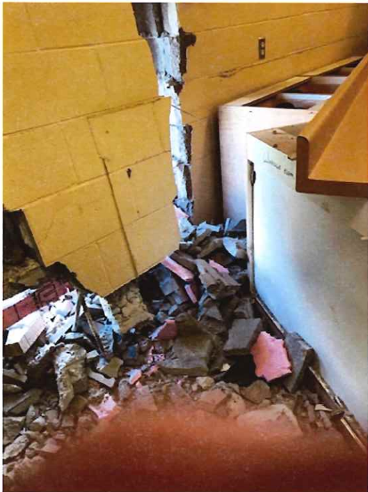
08/10/21- Interior classroom damage
