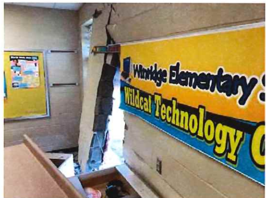
08/10/21- Interior classroom damage
