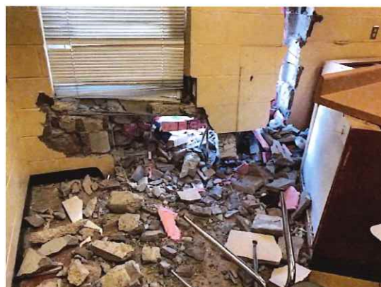
08/10/21- Interior classroom damage
