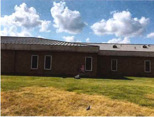
08/10/21- Exterior wall damage from vehicle
