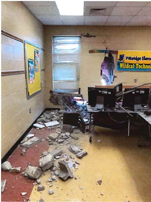
08/10/21- Interior classroom damage
