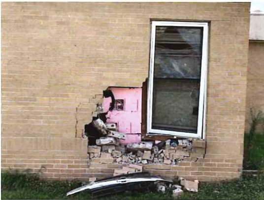
08/10/21- Exterior wall damage from vehicle
