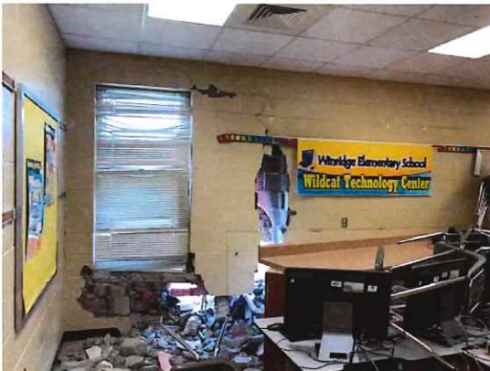
08/10/21- Interior classroom damage
